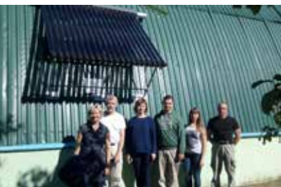
▼ Visiting a solar collector installation at a sport school in Braslav, Belarus.
