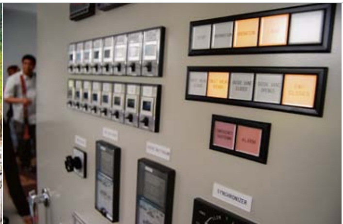
Control panels in the power-generating equipment room
