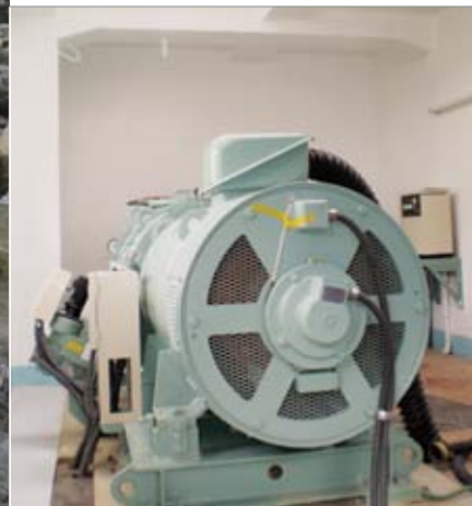
Ambangal 200kW hydro-generating unit
