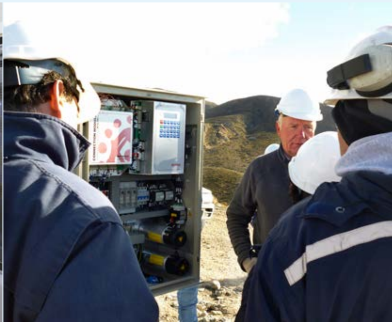
EPEN employees are familiarized with the wind-diesel hybrid system operations on site
