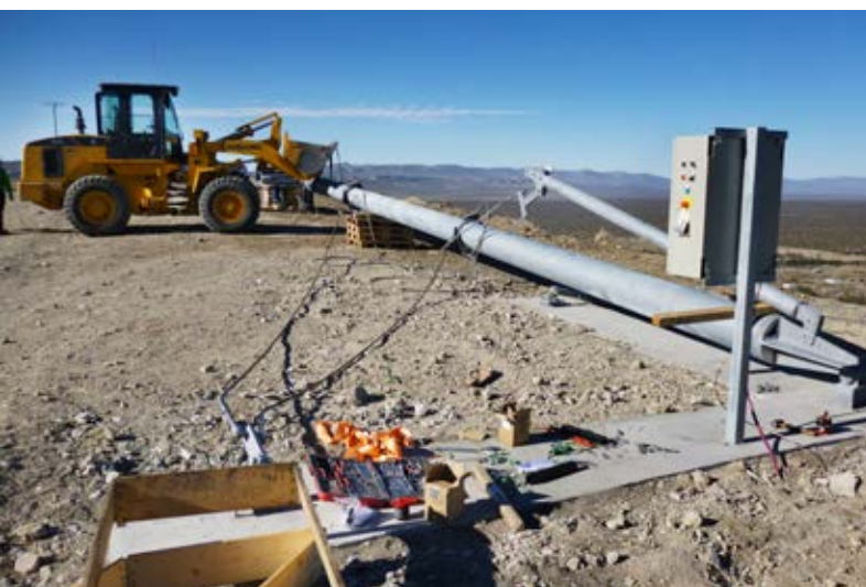
Erection of one of the pole-type guy wired towers in the Chorriaca's wind park
