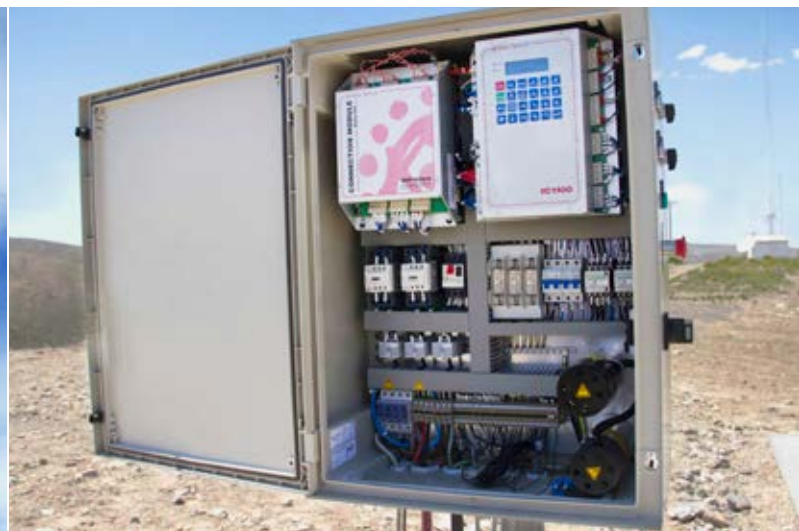
New wind turbine system installed in Chorriaca
