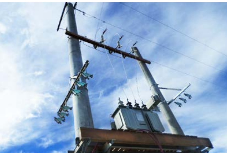
New transmission line built by EPEN to connect the new Cochico power plant to the town
