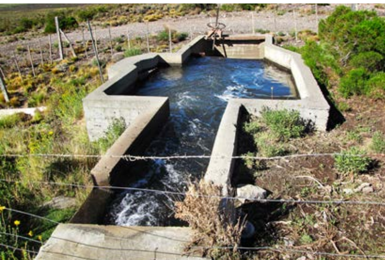
Discharge channel of existing grid-connected mini-hydro plant near Chos Malal
