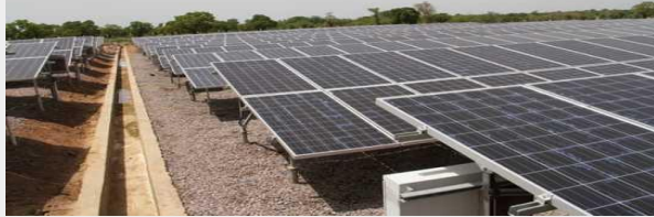
Noguchi Solar Plant
