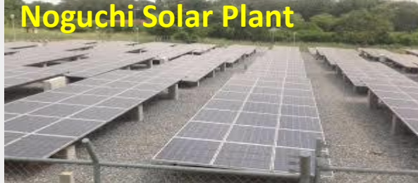
BXC Solar Plant
