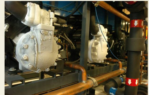
Innovative two-loop refrigeration system
