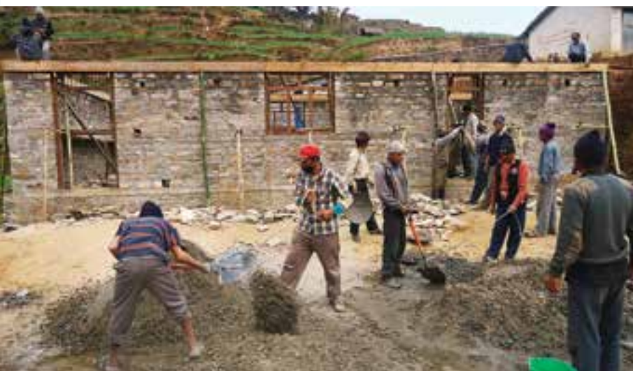
Construction of new computer room and levelling of the childrens' play area
