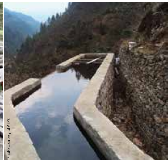
Head tank of a mini-hydropower plant in Nepal installed by AEPC
