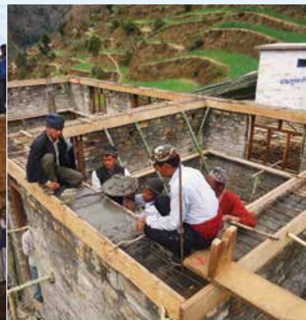
Construction of the new computer room at Malika U Ma Vi School
