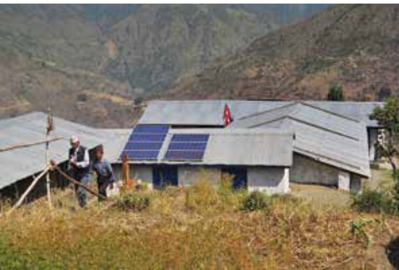
Newly installed PV system at the Rastriya Ma Vi School
