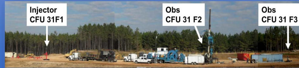
SECARB Demonstration Project in Mississippi
