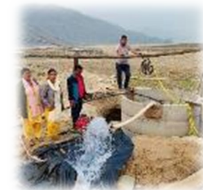
Renewable water lifting system
