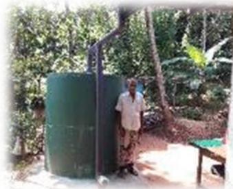
Roof rainwater harvesting.
