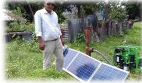
SF2 Solar Water pumps
