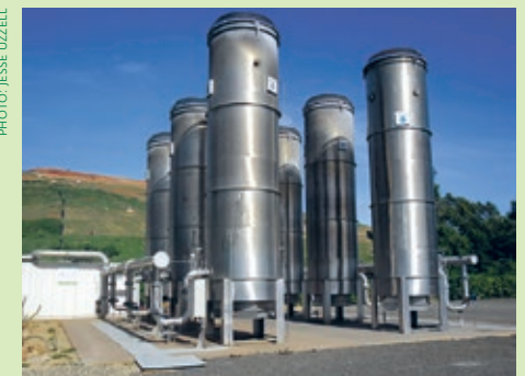
The enclosed flares allow the project to mitigate up to 700,000 tCO 2 e annually.
