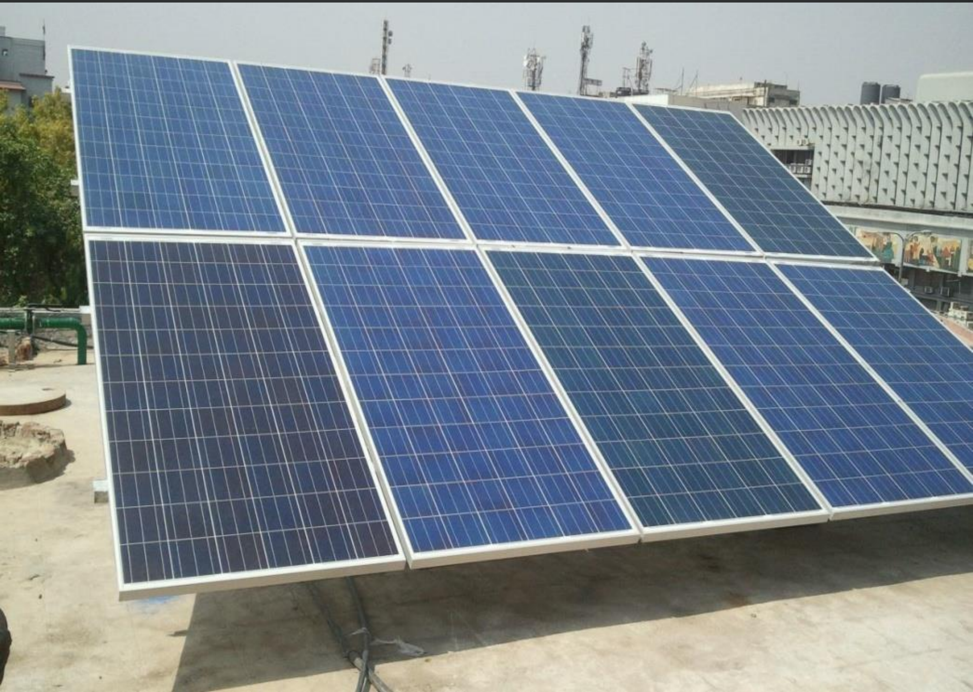
Solar Panel at the rooftop of ITO Station (Underground)
