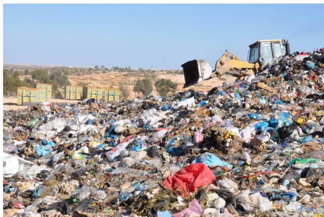
EIB loan helped financing the rehabilitation of an open dumpsite and introducing a sustainable solid waste management system in Tunisia
